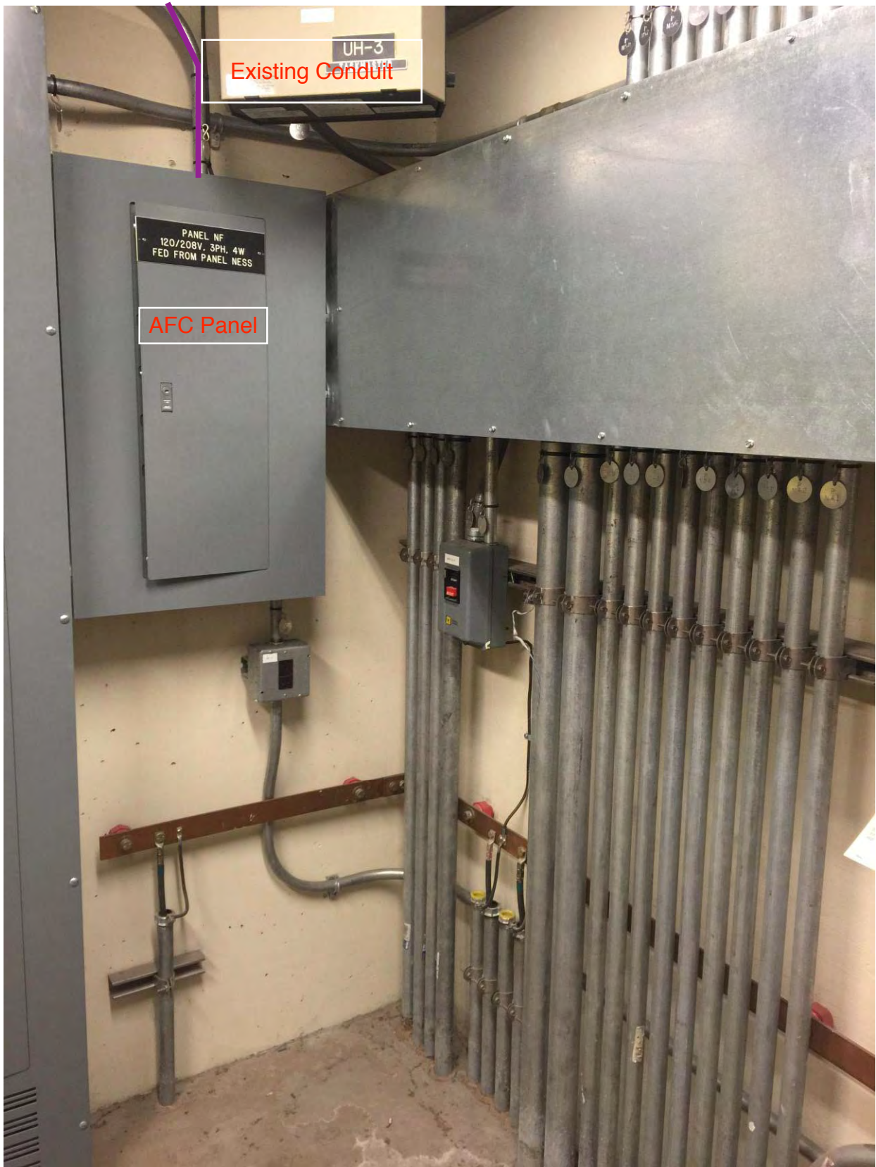
Photo 2 – Existing conduit feeding AFC Panel in Room N201.
